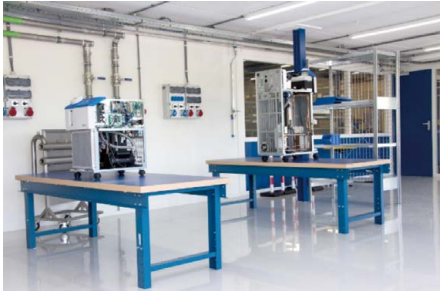
Chiller Repair Center
